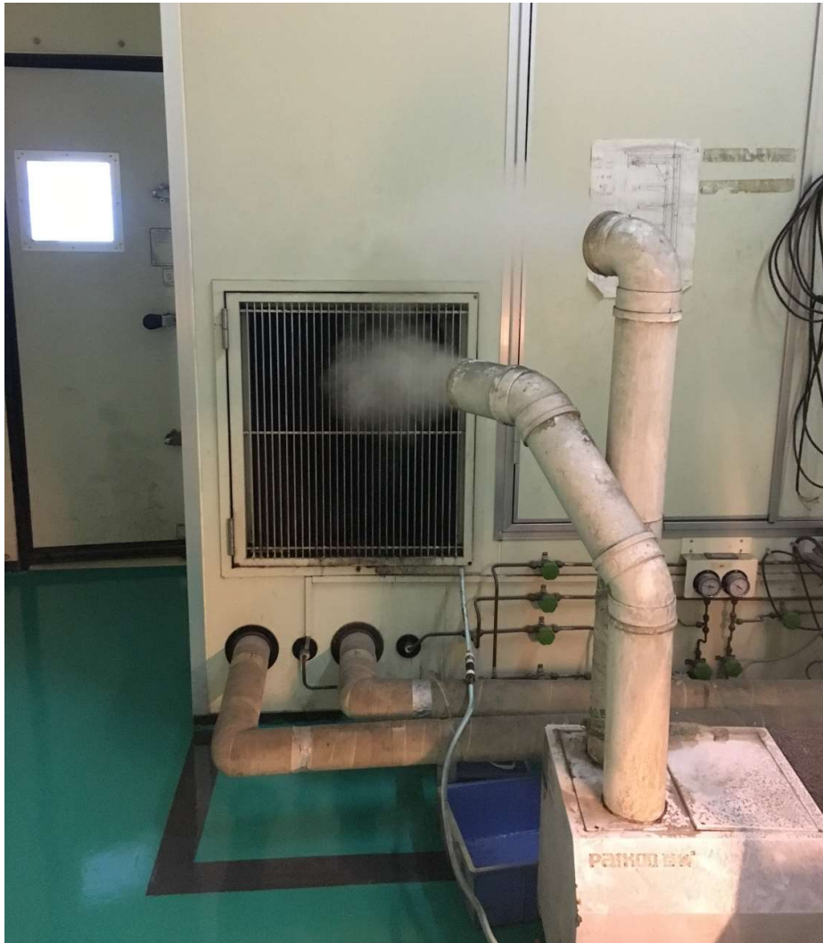
Fig. 1-2 Laboratory air return wall
